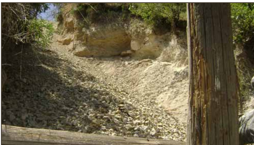
Photo of erosion damage before project began.
