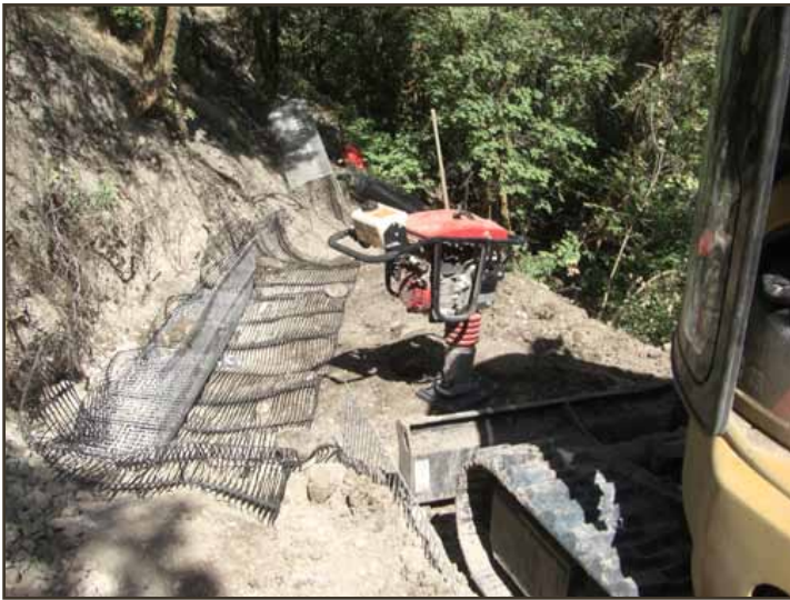
Materials used for stabilization include Gabion baskets, Geo web, compactible soils, gravel mix, top soil and native plant seed.
