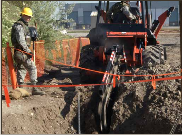
Members of the 130th Engineering Installation Squadron's Cable Team install communications cable during an Operational Readiness Inspection. The 130th Cable Team trenches for the installation of a communications system during the Operational Readiness Inspection.
